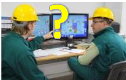
Process operators in the Control Room
